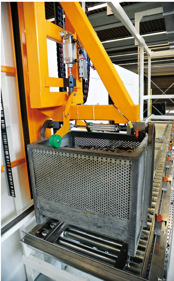
A portal with a special gripper places the basket on the feed conveyor for the machine, installed at a height of around 1.5 metres
